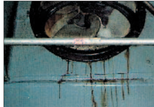
Exhaust fan in need of cleaning
