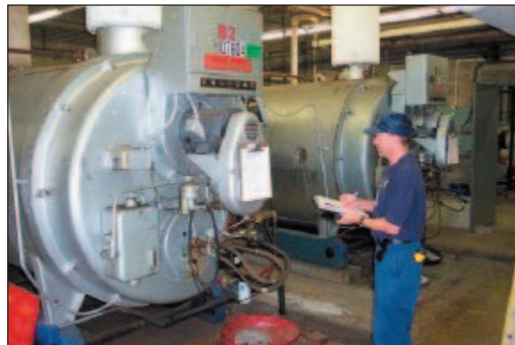
Boiler Inspection under the Boiler Safety Act
