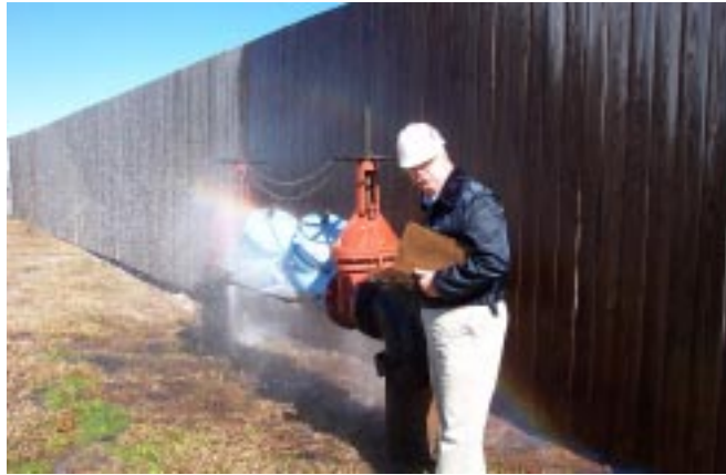
SFM Fire Protection Specialist, Z.K. Roberts inspects freeze damaged water main supplying fire sprinkler system
