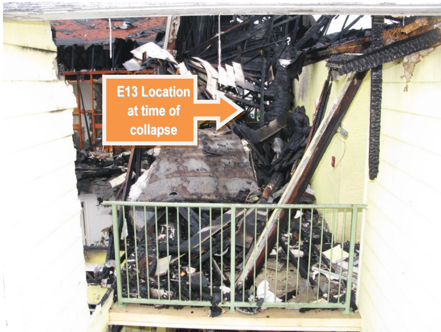
Picture 6 –View from Side A of 3 rd floor landing on Side B stairwell.
