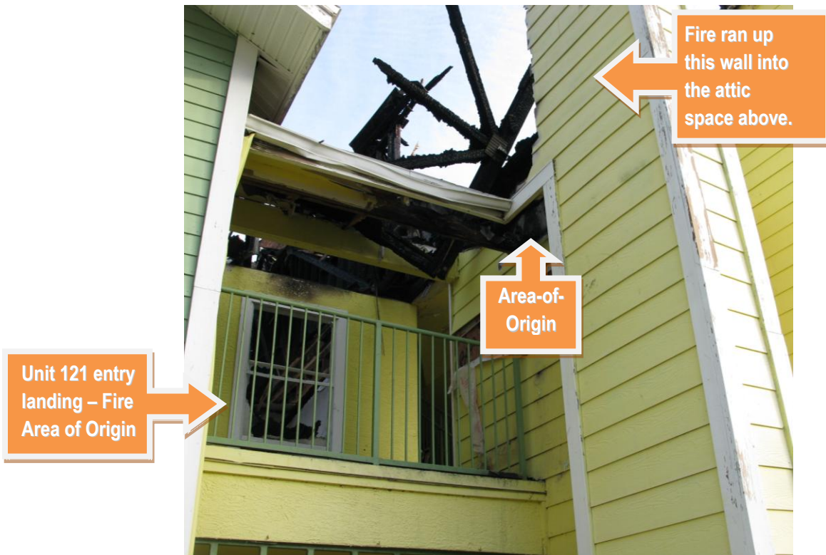
Picture 8 – Unit 121 2 nd floor entry landing indicating the area of fire origin and route of travel up exterior wall to the attic above.
